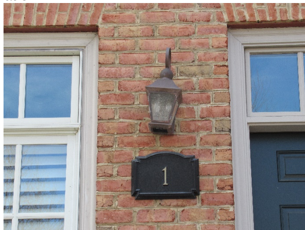
Tilted light fixture
