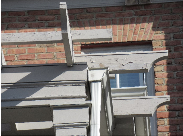
Finish deterioration, shown at Unit 4
