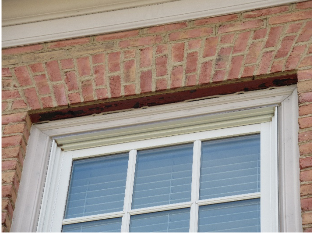
Lintel finish deterioration, shown at Unit 3
