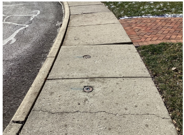
Cracks and settlement
