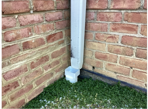
Misaligned downspout, shown at Unit 10
