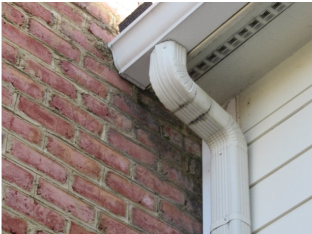
Evidence of leakage at the seams
