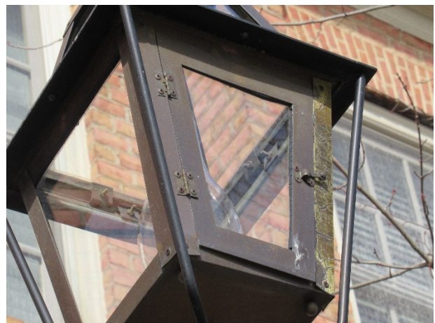
Finish deterioration, shown at Unit 7
