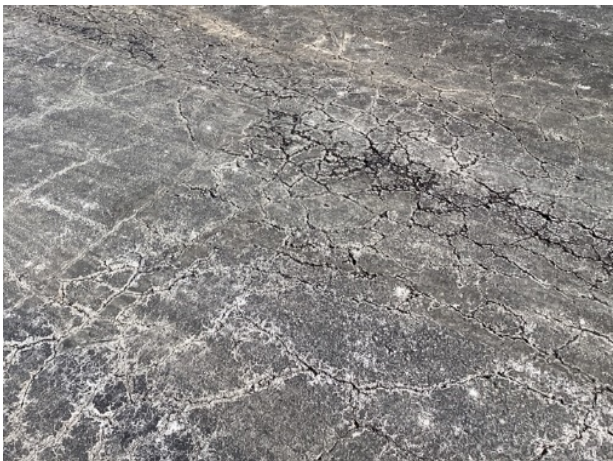
Alligator cracks and surface deterioration
