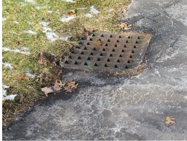
Catch basin – note settlement
