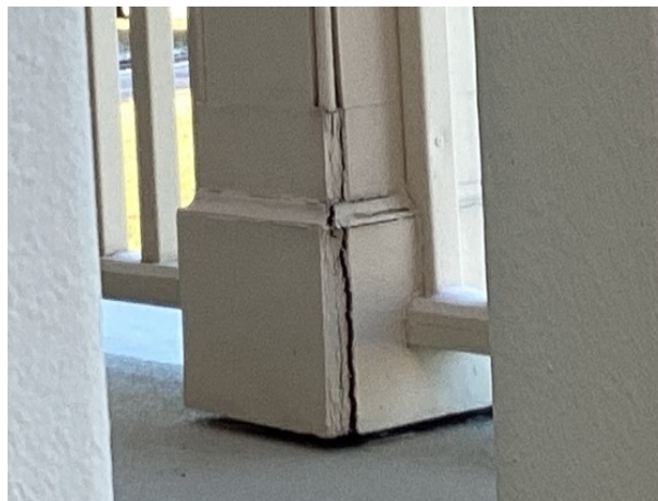
Wood split and finish cracks, shown at Unit 9
