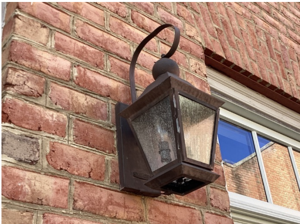
Light fixture at Units 1-9 – note finish deterioration
