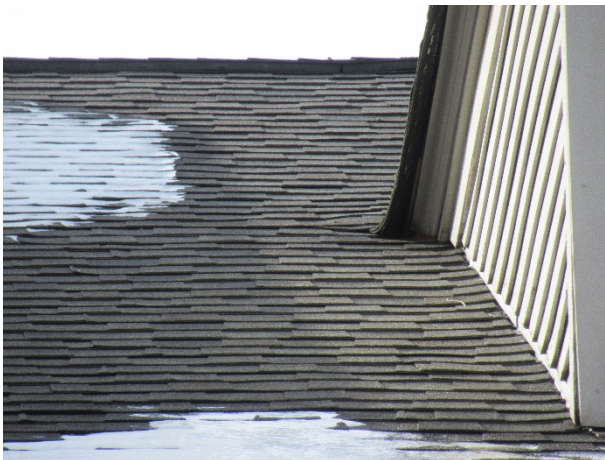
Shingle lift and deflection, shown at Unit 3
