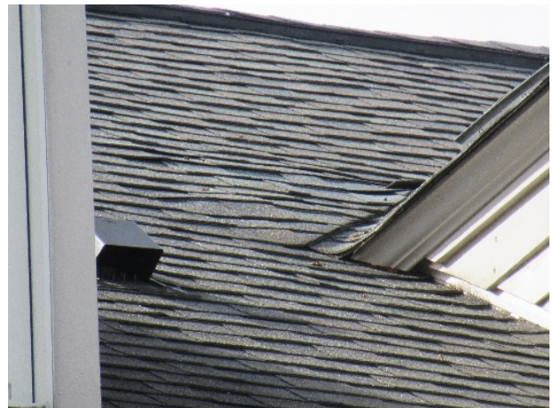
Sheathing deflection, shown at Unit 4
