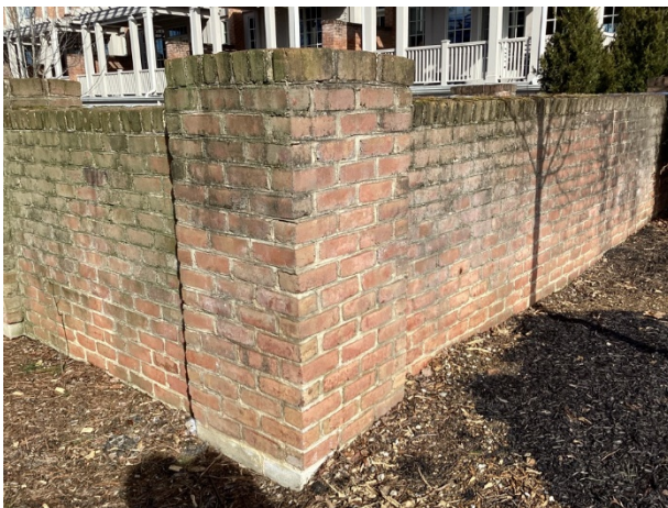
Organic growth and mortar loss at retaining wall
