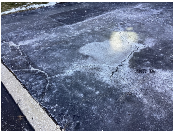
Cracks, surface wear and previous patching at Unit 9 driveway
