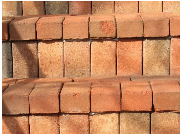
Damaged bricks, shown at Unit 7
