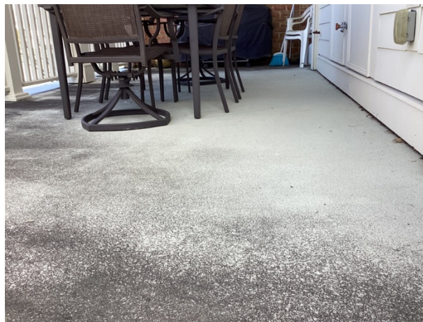
Deteriorated concrete coating
