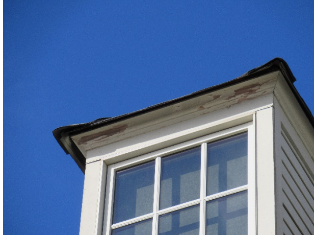
Paint finish deterioration
