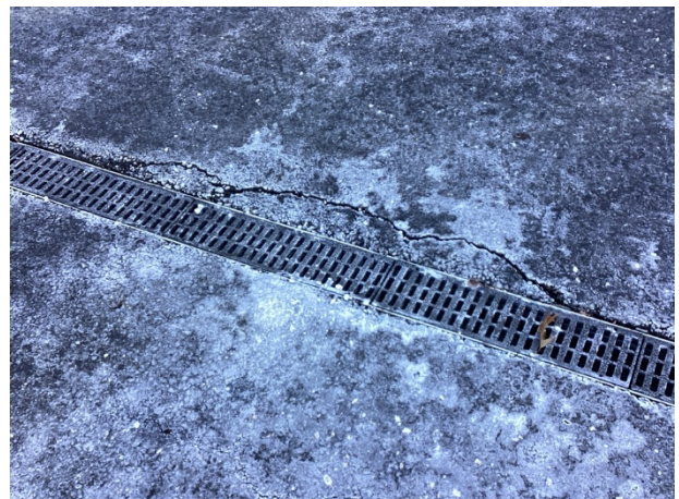
Cracks at Unit 12 driveway
