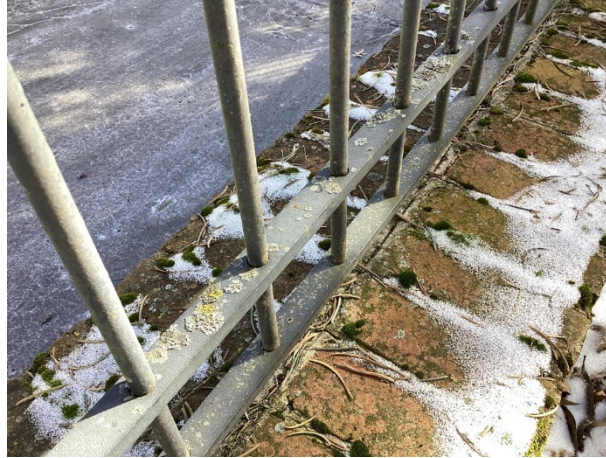
Finish deterioration and organic growth
