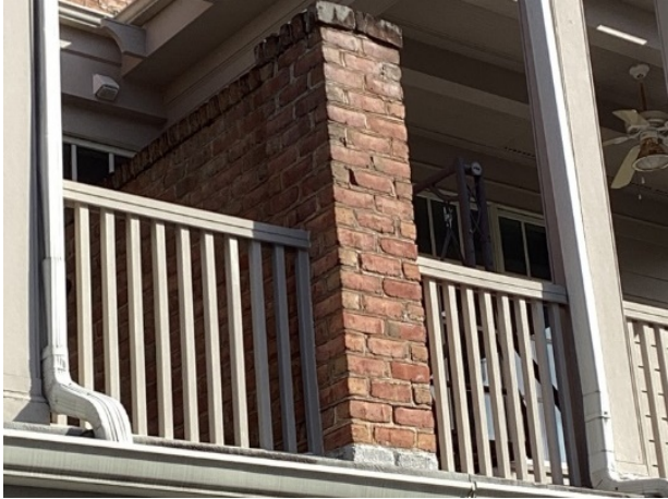
Mortar loss at privacy wall between Units 2 and 3
