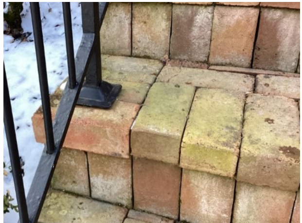
Efflorescence and organic growth, shown at Unit 5
