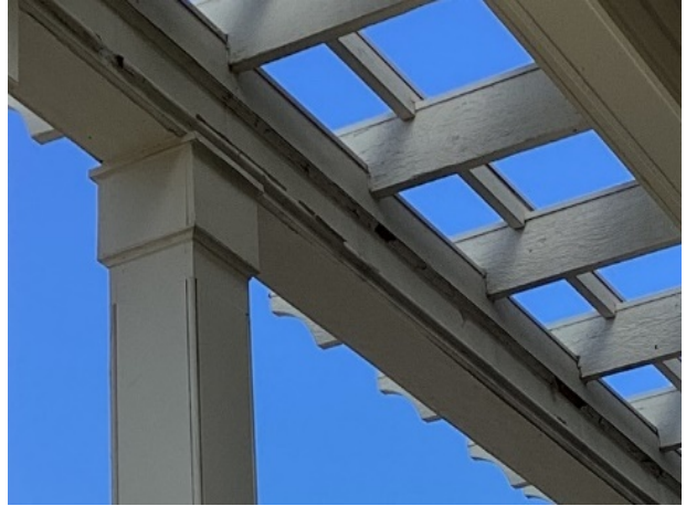
Wood split and finish deterioration, shown at Unit 6
