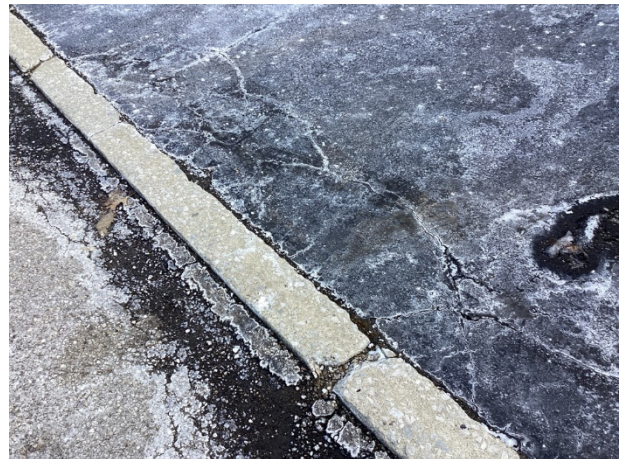
Settlement and cracks at Unit 7 driveway
