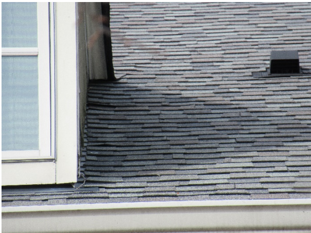
Shingle lift and deflection, shown at Unit 8
