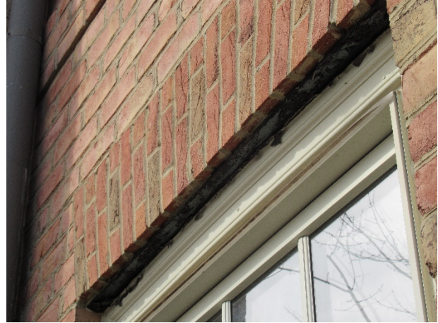
Lintel finish deterioration, shown at Unit 9
