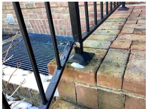
Damaged railing, shown at Unit 1
