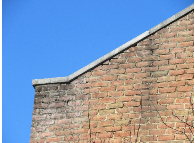
Mortar loss and staining
