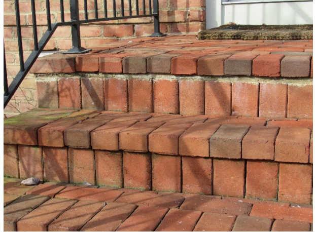
Evidence of previous repairs, shown at Unit 9
