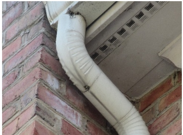
Evidence of leakage
