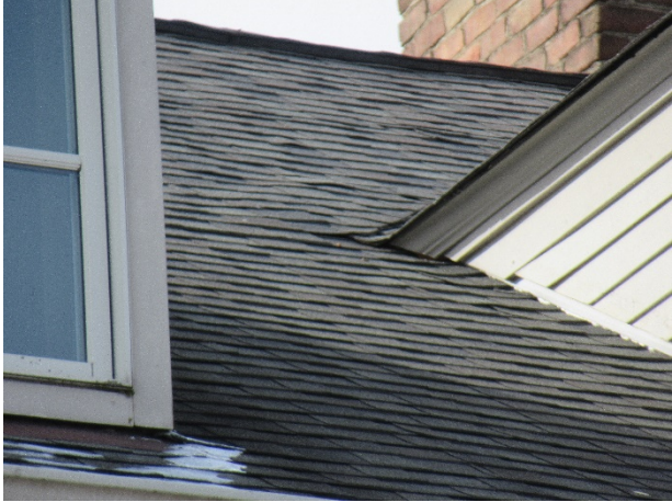
Shingle lift and deflection, shown at Unit 5
