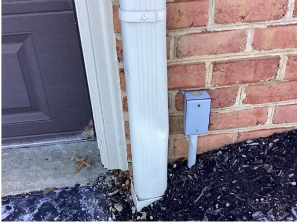
Downspout dent, shown at Unit 9
