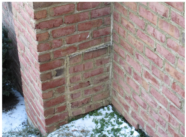
Evidence of previous repairs
