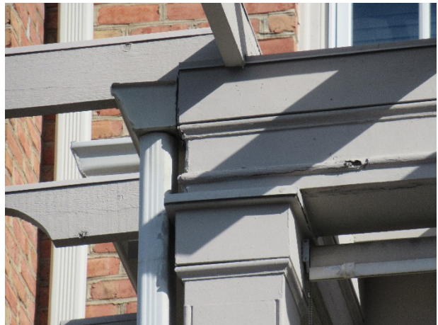
Pergola damage, shown at Unit 3
