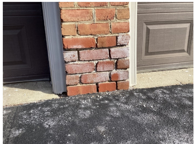
Mortar loss, shown at Unit 3
